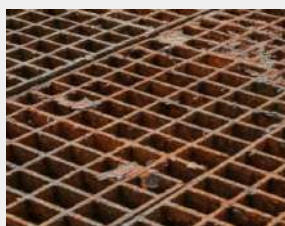
Discoloration and Corrosion
